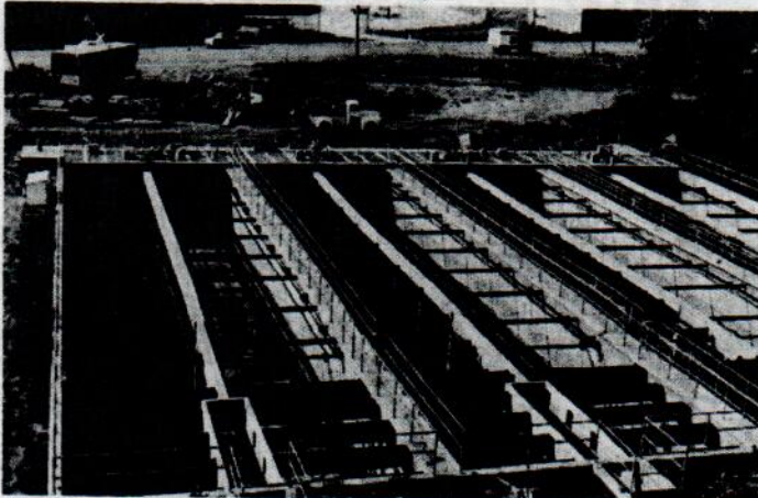
Shown in the photo are the three new digesters, which have been completed at Davenport's expanded sewage treatment plant on South Howell Street. (Staff Photo)
